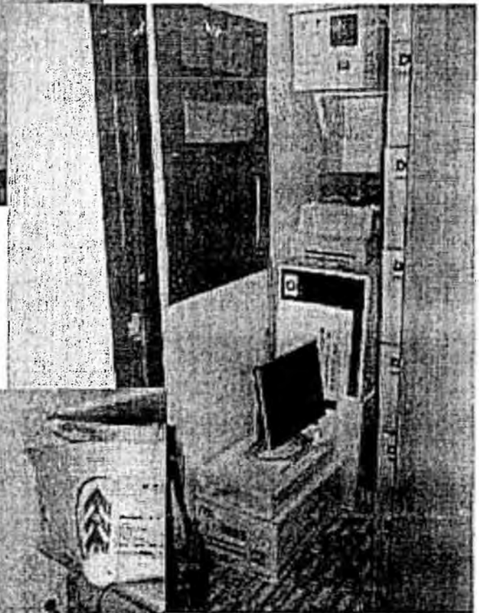
Blocked Electrical Panel
