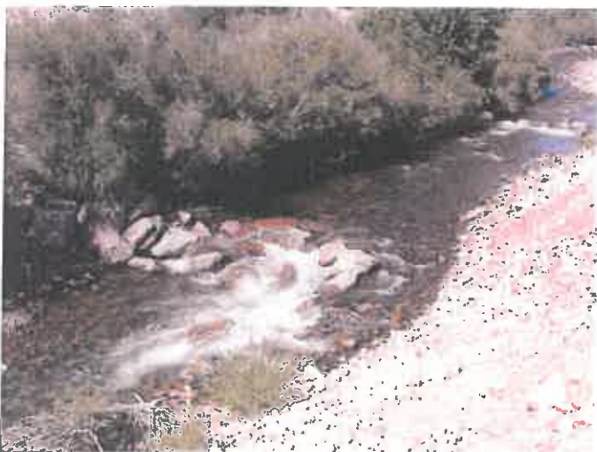
Existing damaged drop structure along the river
